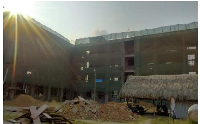
Fencing for works for occupational safety and environment around the construction area
